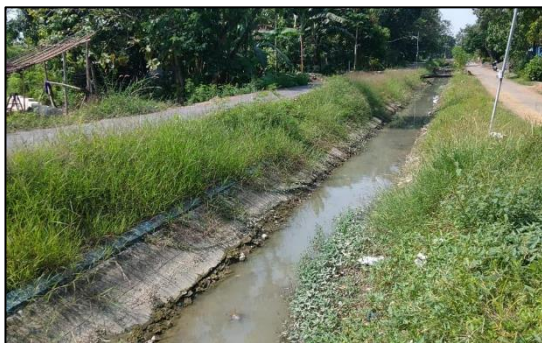
Fig. 4. Existing Condition Hm 58+00
