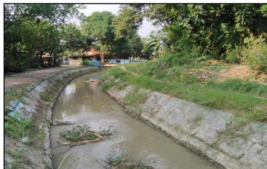
Fig. 5. Existing Condition Hm 71+00
