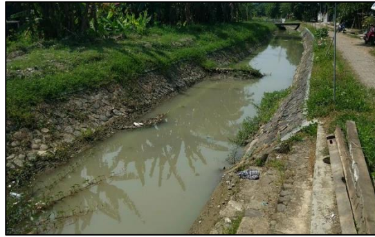
Fig. 3. Existing Condition Hm 50+00
